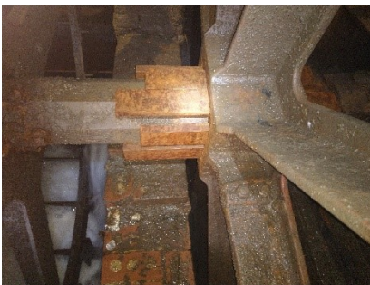
Figure 2 Job Completed. Wedges left log pending future repair work to adjacent structure
